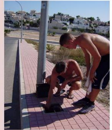
Sean from Omega Electrics with apprentice look down into the murky world of cables and dirt!
